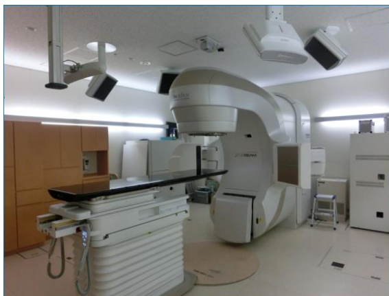
Example of delivered system (Uonuma Kikan Hospital)
