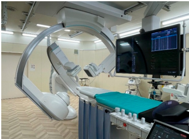
Fig. 3 The Trinias Opera system installed in January 2025
